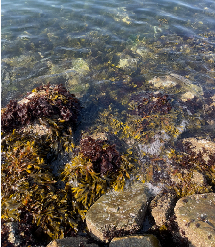
Figure 12: Additional photo of the rocks supporting the seawall that is submerged under water during high tide and presents with seaweed and barnacle growth.
